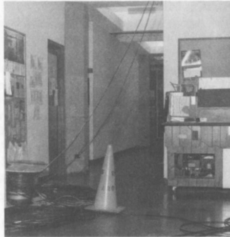
All the wire in the hallway may seem unsightly, but it's the harbinger of good times at GSU because it means a new telephone system is close to reality at last. Many new communication features will be available once the installation process is completed.
