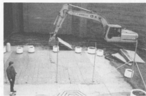
A crane lifts sections of the patio as site preparation begins for The Regional Center for Technology and the Performing Arts. Construction work is expected to take two years.
